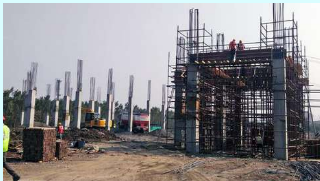
The construction site of hydrazine hydrate plant at Gujarat Alkalies & Chemicals Limited in Dahej. File | Photo Credit: Special arrangement
